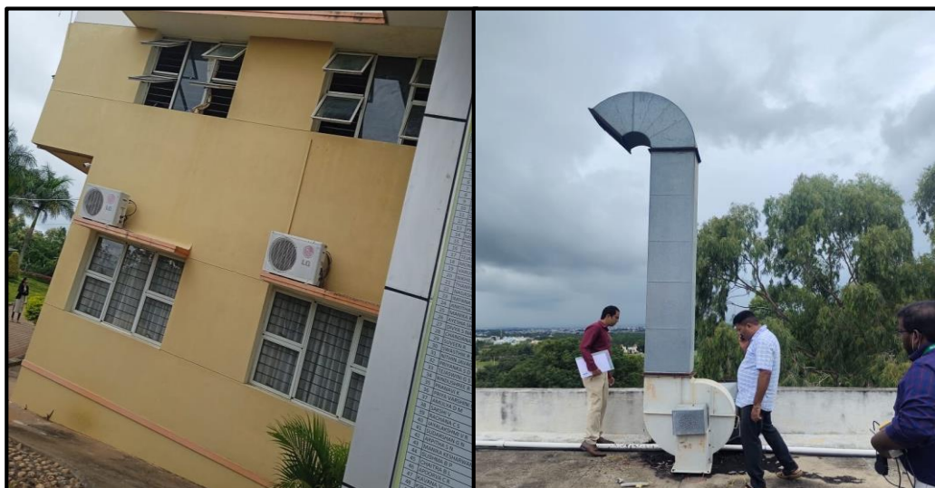
Ventilation and Exhaust system Facilities in AIT Buildings
